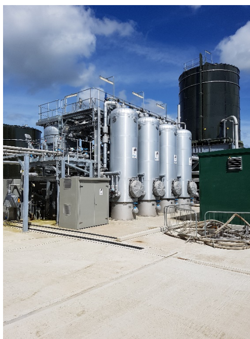
Cambi's Plant at Basingstoke, England. Photo: Cambi
