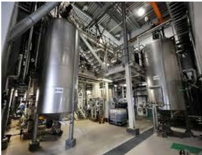
Photo showing Borregaard's Demo Unit in Sarpsborg, which were used to showcase faster and more complete saccharification of Borregaard's BALI-pretreated spruce feedstock at demonstration scale.
