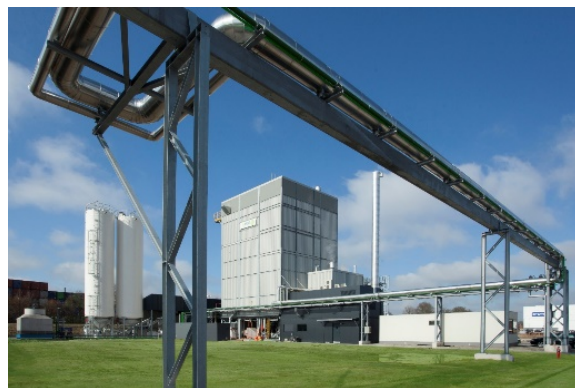
The Empyro plant in Hengelo (NL) (photo: BTG).
